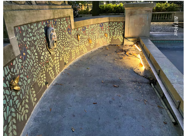
Fountain Lights - One Out.
