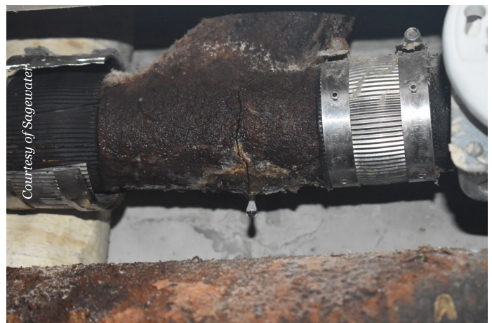
Hidden leaks can be needlessly costly.
